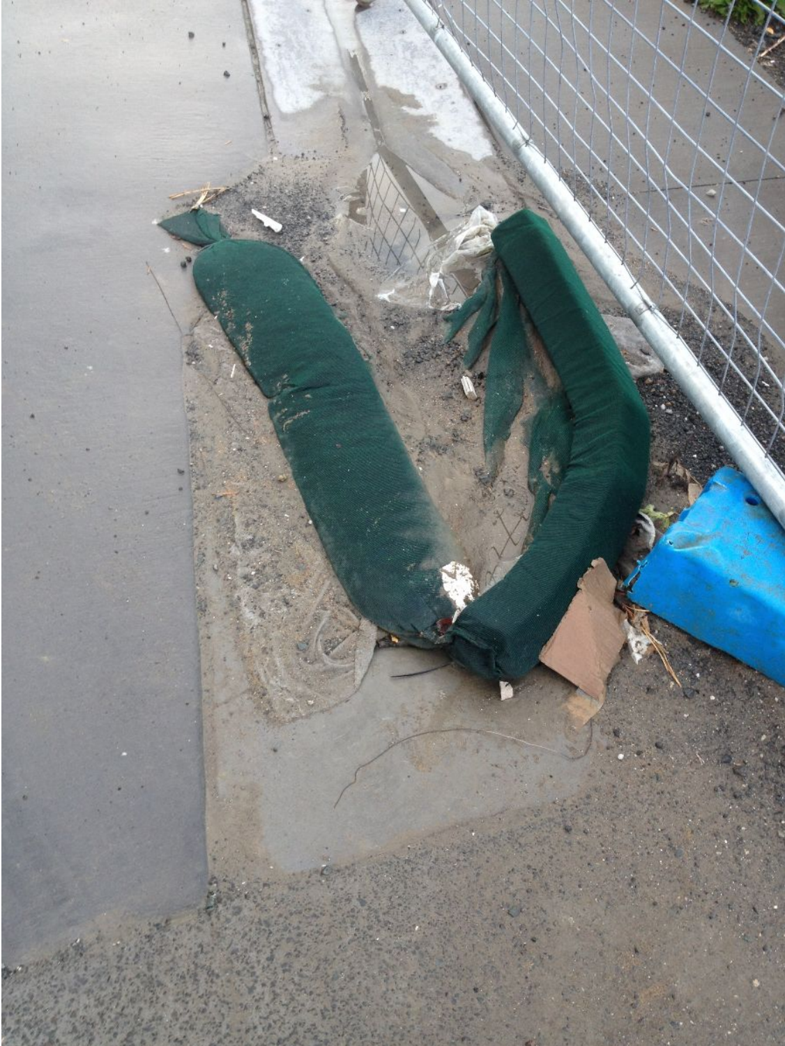
Unmaintained sediment control at catchpit on Lalanga Lane development, Glen Innes. Photo credit: Beth Evans
